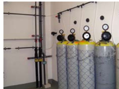
Chlorine bottles with mounted chlorinator C2213
