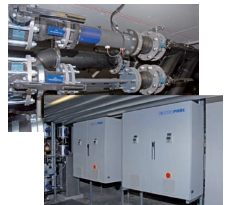
The Technopool electrolysis system
