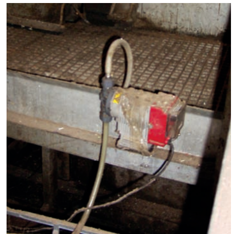
Image 2: Dosing pump in a plastics recycling plant
