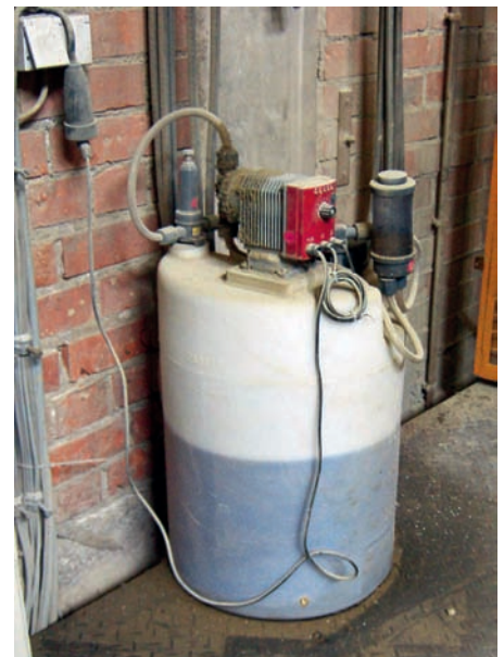
Image 1: Dosing station in a brickyard
